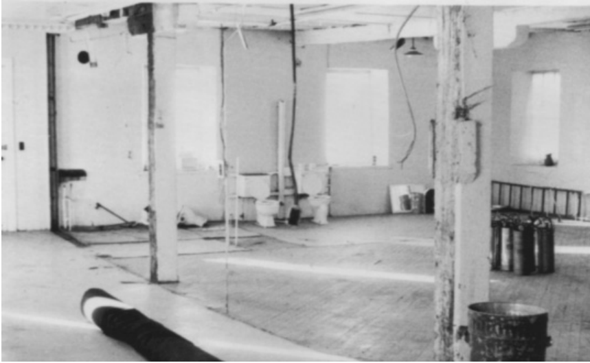
1972-1973 The Wandermeer Lounge in the winter of 1972-1973. While the outside crews were busy with pile driving and dock construction, the inside crews plastered the walls, leveled the floors, rewired the building, and created two large and more private washrooms. A kitchen completed the upstairs renovations.
