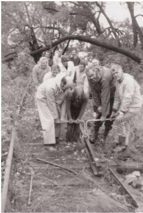
1973 Removal of old rail line to make way for the club. Photo Credit: Tom Stubbs
